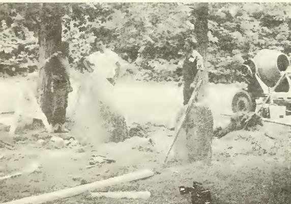
DPW workers set Town of Rye Stone for Dedication on Olde Home Days.
